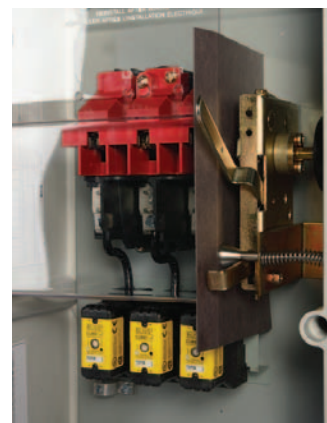
Enhanced Line Shield and Interlock Defeater
